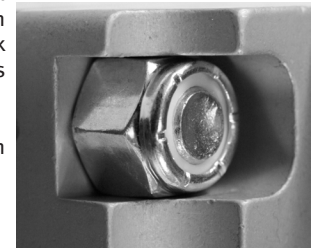
Fig 21 Bolt protrudes just beyond flush
